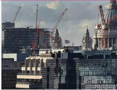
London's mayor Sadiq Khan has said he intends to fine construction firms over air quality.
