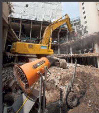
DustBoss spraying mist at South Bank Tower
