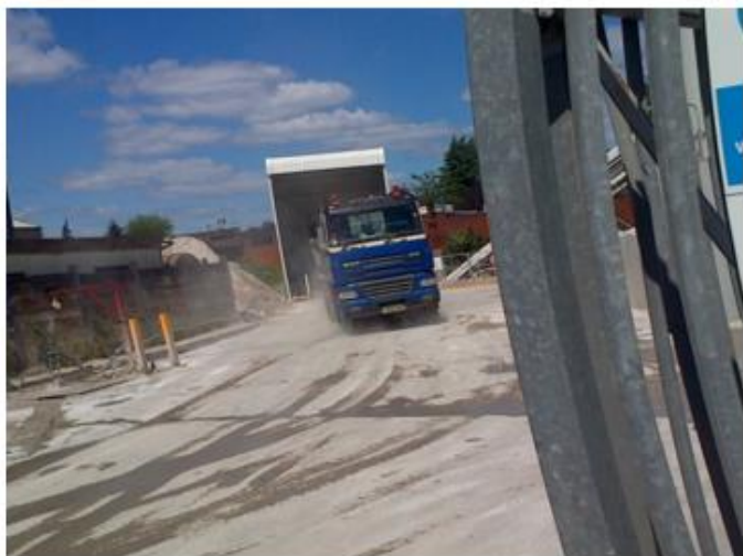
Dust blown up by lorry manoeuvring at western
